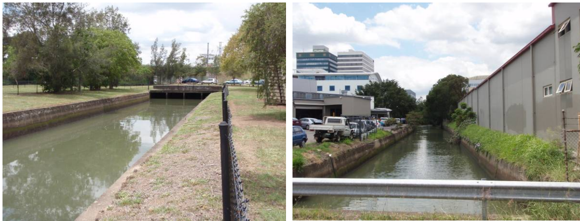
■ Figure 2 :Open concrete-lined tidal drainage channels downstream of the study corridor at Milton Park and Kilroe Street prior to discharge into the Milton Reach of the Brisbane River
